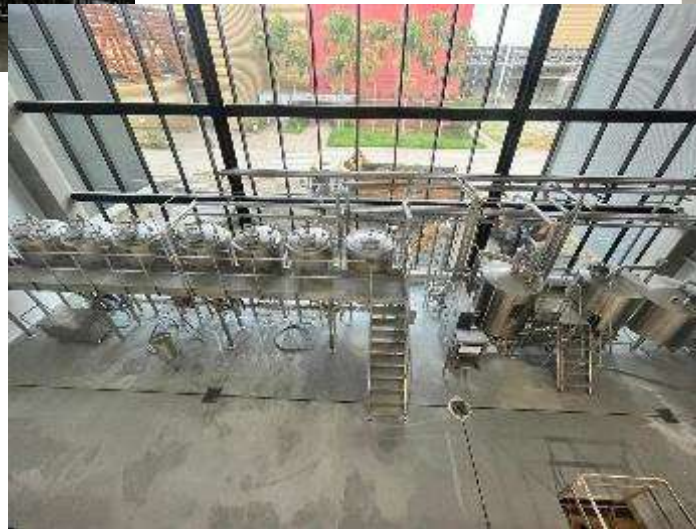
PILOT PLANT – VIEW FROM BAR
